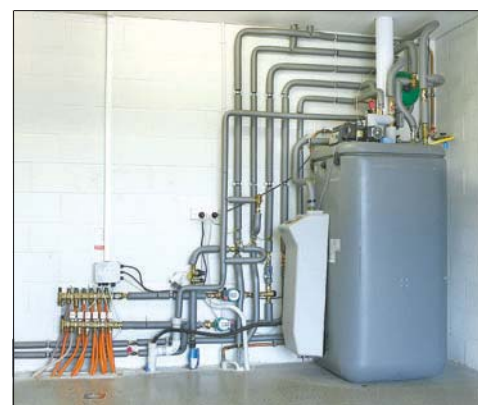
Even the boiler is state of the art — an integrated gas and solar one from Germany.
